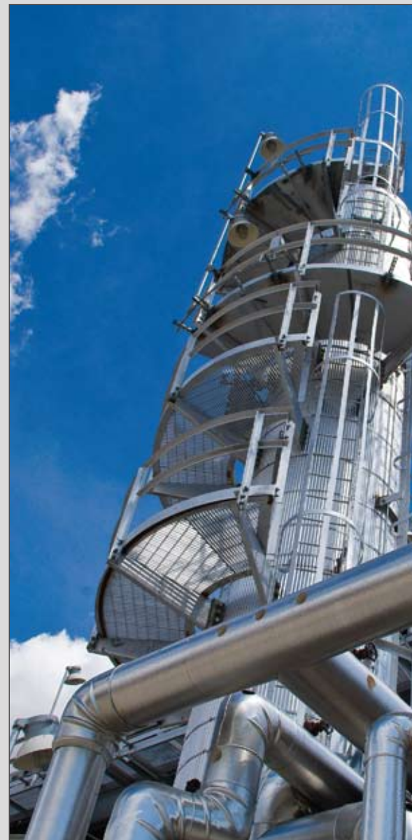
Navajo Refinery Company, L.P., Inc., a subsidiary of Holly Corporation selected this ROSE unit for their Artesia, New Mexico refinery.
